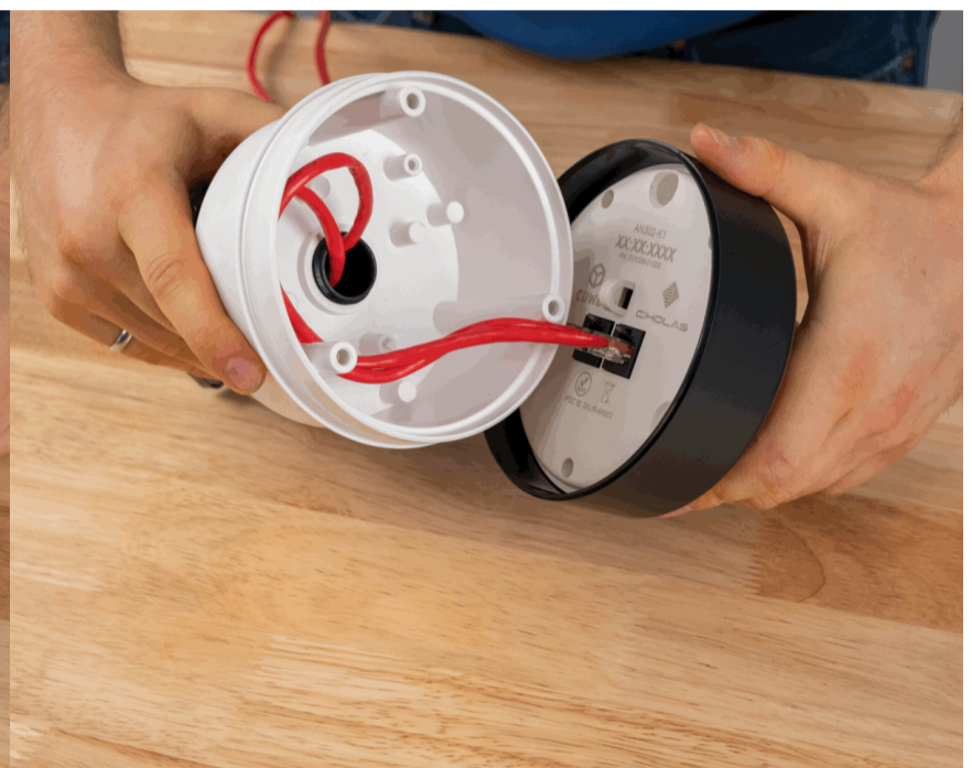
View of service loop
